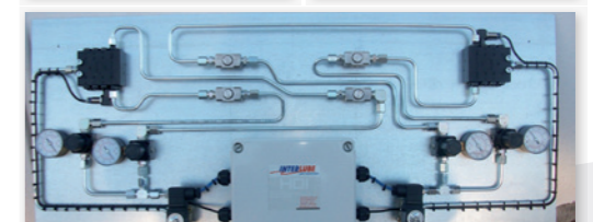
Grease Spray Systems
